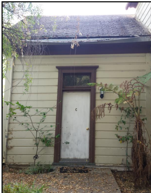
Close up of (N) entrance to office addition on E side of residence. It retains original siding, door frame and transom with inappropriate replacement door; roof and foundation damage, photo view toward S, 12/2017.
