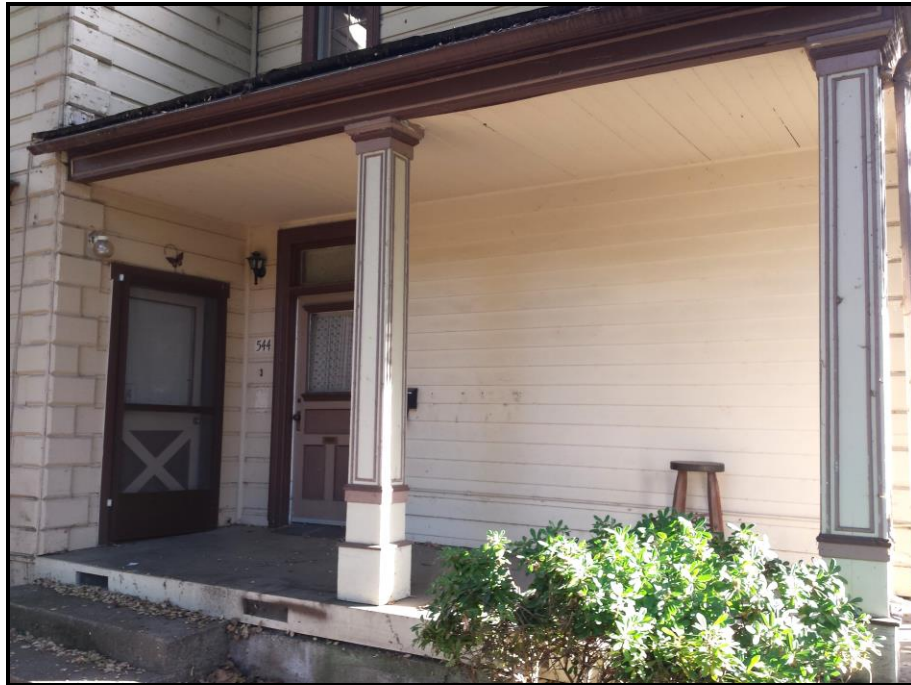
Front porch shows major alterations in design and materials after conversion to apartments and subsequent fire damage; photo view toward SE, 12/2017
