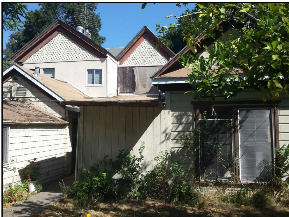
S elevation shows a deteriorated hodgepodge of additions, photo view toward NE, 12/2017.
